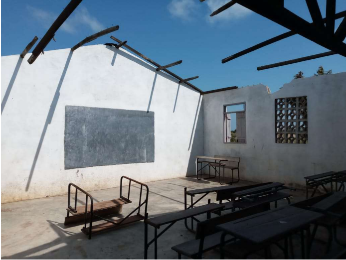
Fig. 3 EPC Nhahole with 4 classrooms and 1 administrative room damage by cyclone Idai
